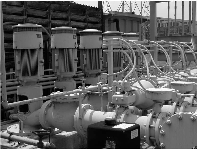
Figure 6.22 Maintenance and repair is a significant component of pumping system life-cycle costs, and an effective maintenance program can minimize these costs. (Courtesy of, and with joint permission of the Hydraulic Institute, Parsippany, NJ; Europump, Brussels, Belgium; and the U.S. Department of Energy Office of Industrial Technologies, Washington, D.C.)
